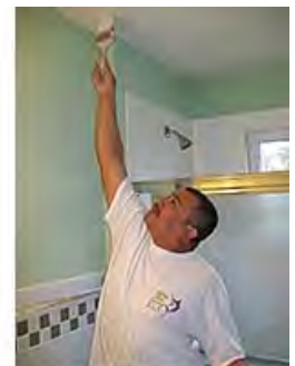
Builder Captain Madison Homes, Inc., worked closely with five trade partners on the renovation.
